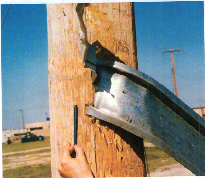
Figure 1 Tornado Damage in Kansas The force of the wind during a tornado was strong enough to drive a piece of metal into the utility pole.
